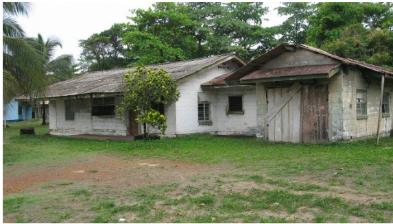
House at ELWA in need of restoration
